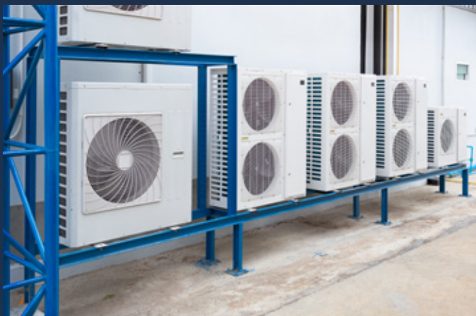
REFRIGERATED AIR HANDLER / CONDENSING UNITS
